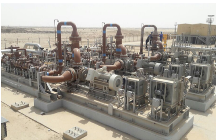
Figure 3. Large gathering system with multiphase pumps.
