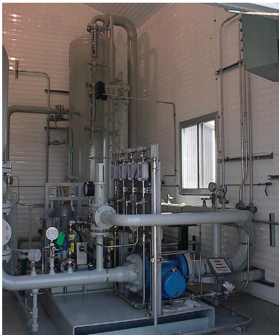
Devon Canada's multiphase pump installation employs a free-water knockout to catch produced liquids, which enables the pump to run on 100 percent gas for extended periods.
