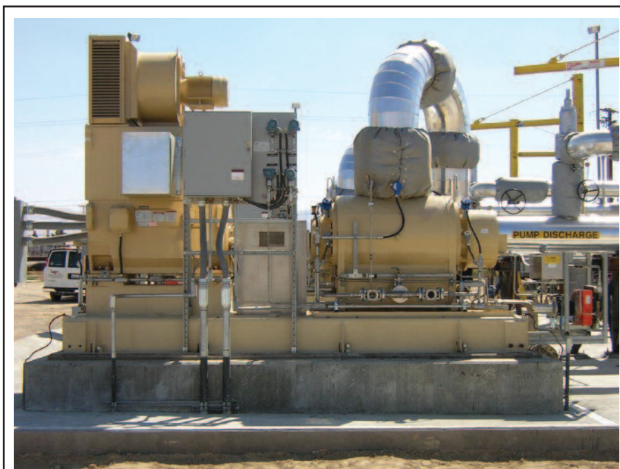
Multiphase pumping offers the unique ability to boost both gas and liquids in a single process with a single piece of machinery in both onshore and offshore applications. Shown here is a typical multiphase pumping unit in on onshore installation.
